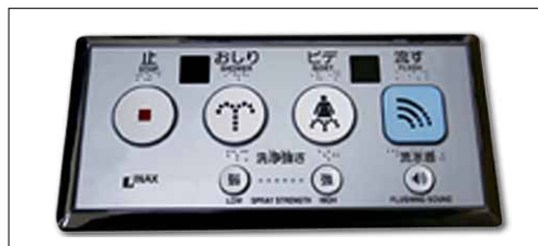
Control panel for public toilet
